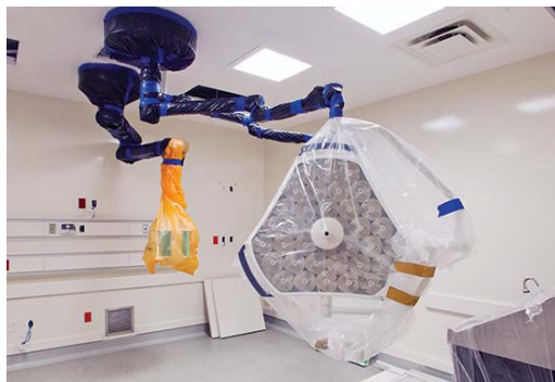
Lighting in Emergency Department resuscitation room
