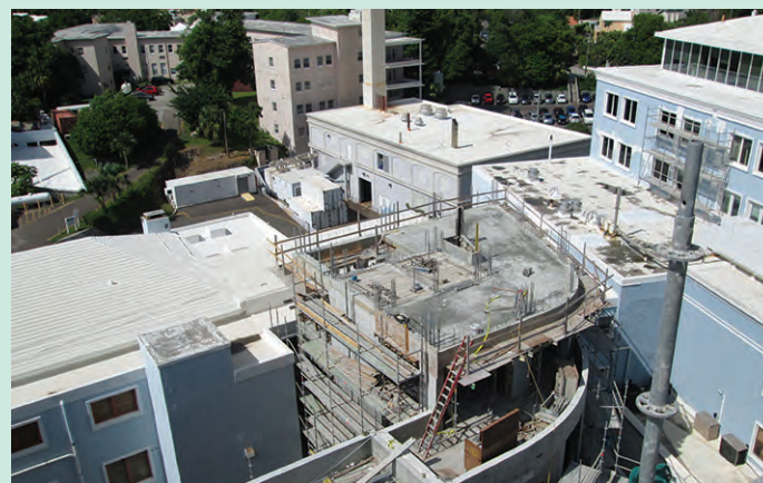
Concrete slab works on level 3 of the building linking the Acute Care Wing to the existing KEMH.
